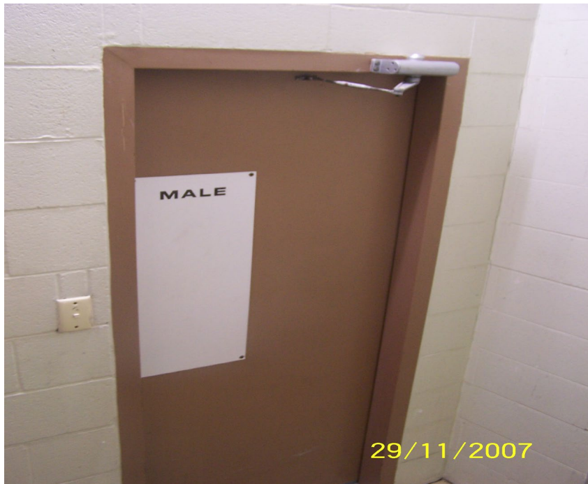
All Levels - Photo No: 76 Gents Toilet – Door (Fire)
